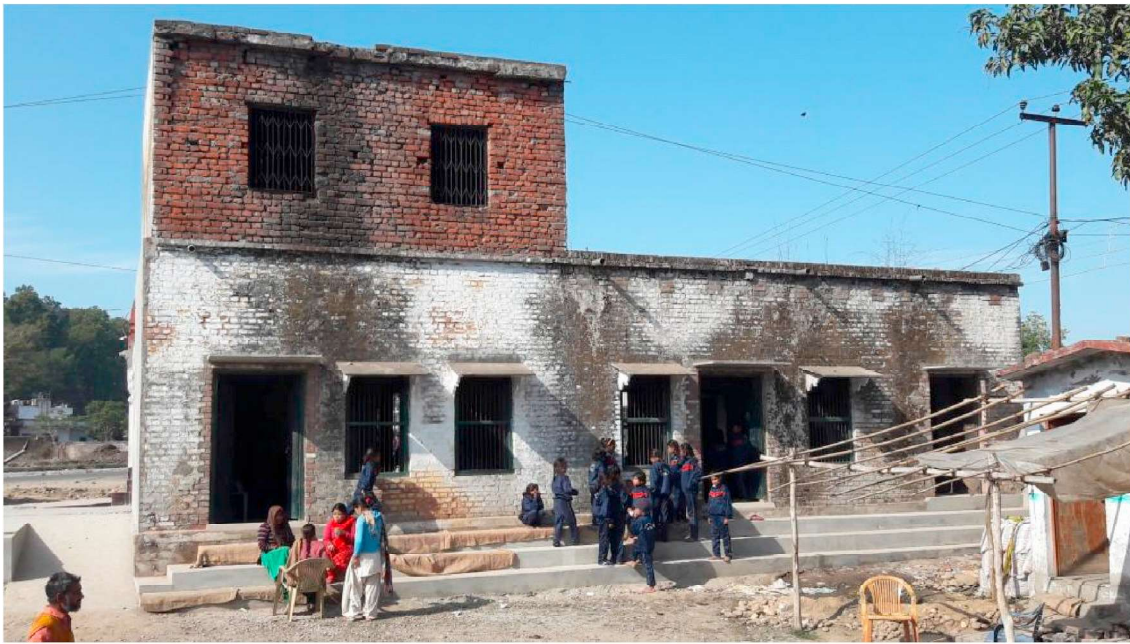
Fig. 8. Primary School at Motichoor in Dehradun representing a non-engineered double storeyed masonry structure.
