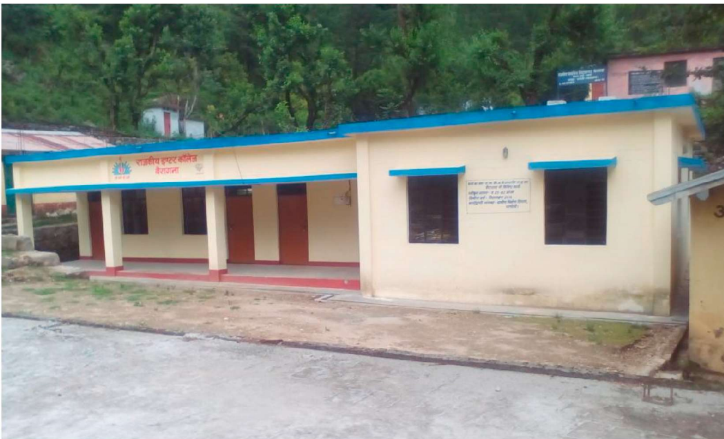
Fig. 12. Single storeyed Government Inter Collage at Bairangana in Chamoli district having RCC slab as the roofing material and exhibiting re-entrant corner.
