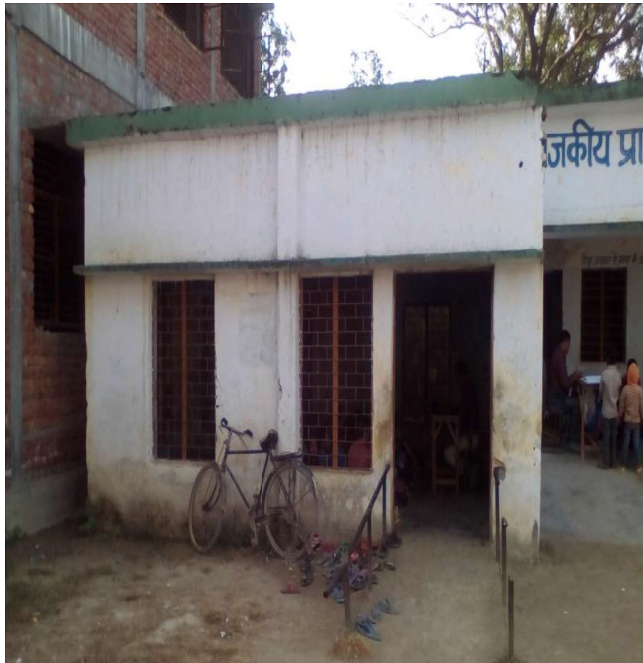
Fig. 14. Government Primary School at Bajpur in Udham Singh Nagar district; vulnerable to pounding during seismic shaking.
