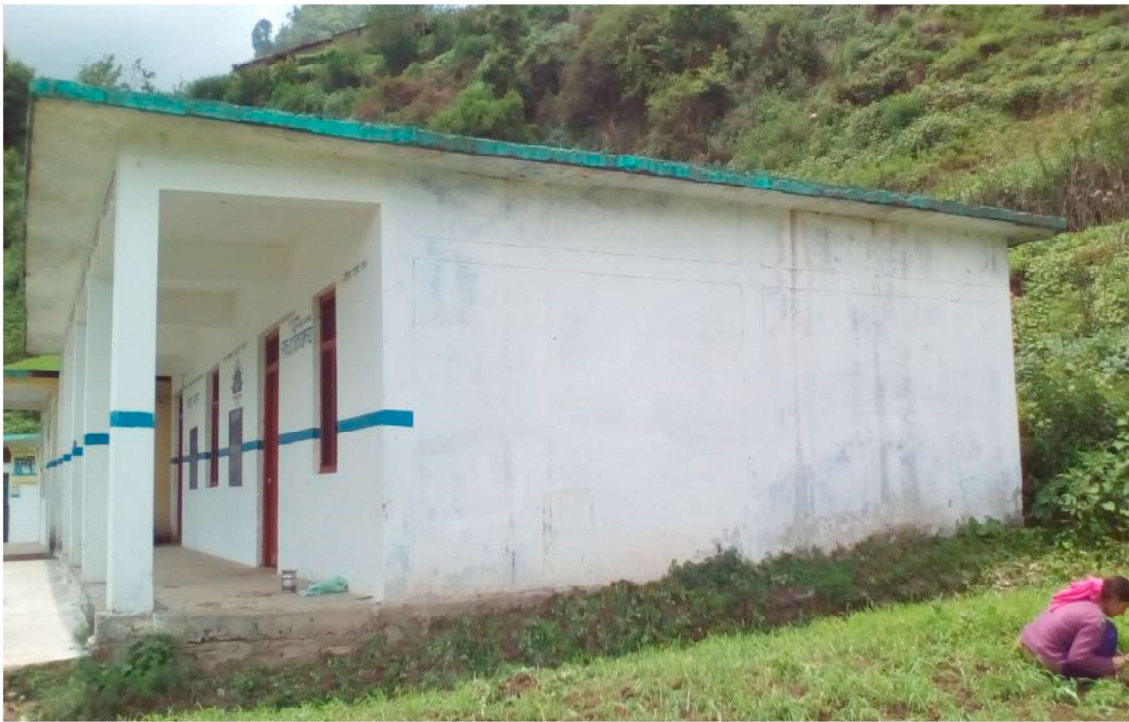
Fig. 6. Government Inter Collage at Trijugi Narayan in Rudraprayag district having RCC slab as the roof and built over soft soil.
