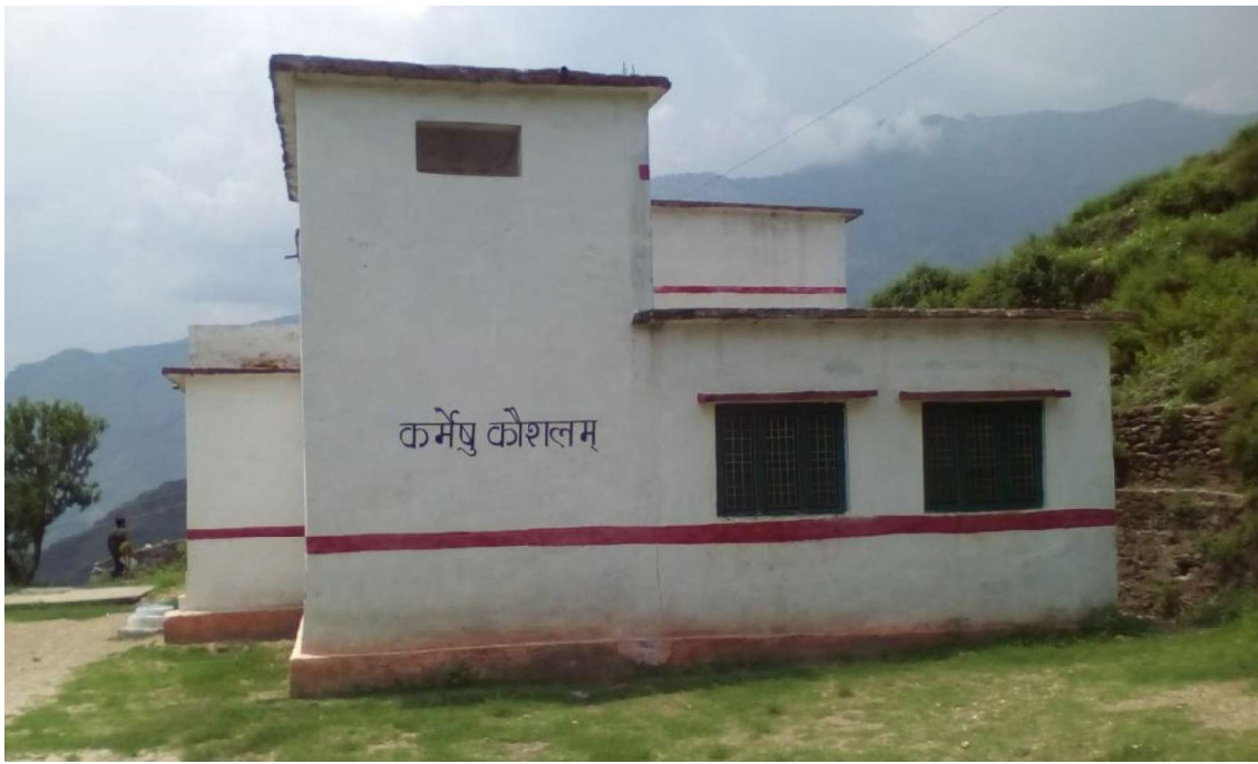
Fig. 13. Re-entrant corners in Upper Primary School at Balidhar in Chamoli district.
