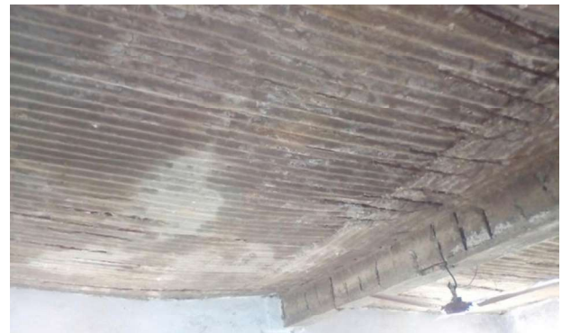
Fig. 5. Poorly constructed roof with clearly visible reinforcement at Government Primary School Mhalchora in Bageshwar district.
