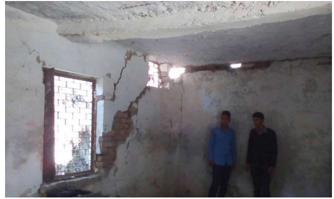
Fig. 4. Wide shear cracks in masonry wall of Government Inter College, Pitrdhar (Rudraprayag district) together with poorly constructed beam of non-uniform shape showing deflection.
